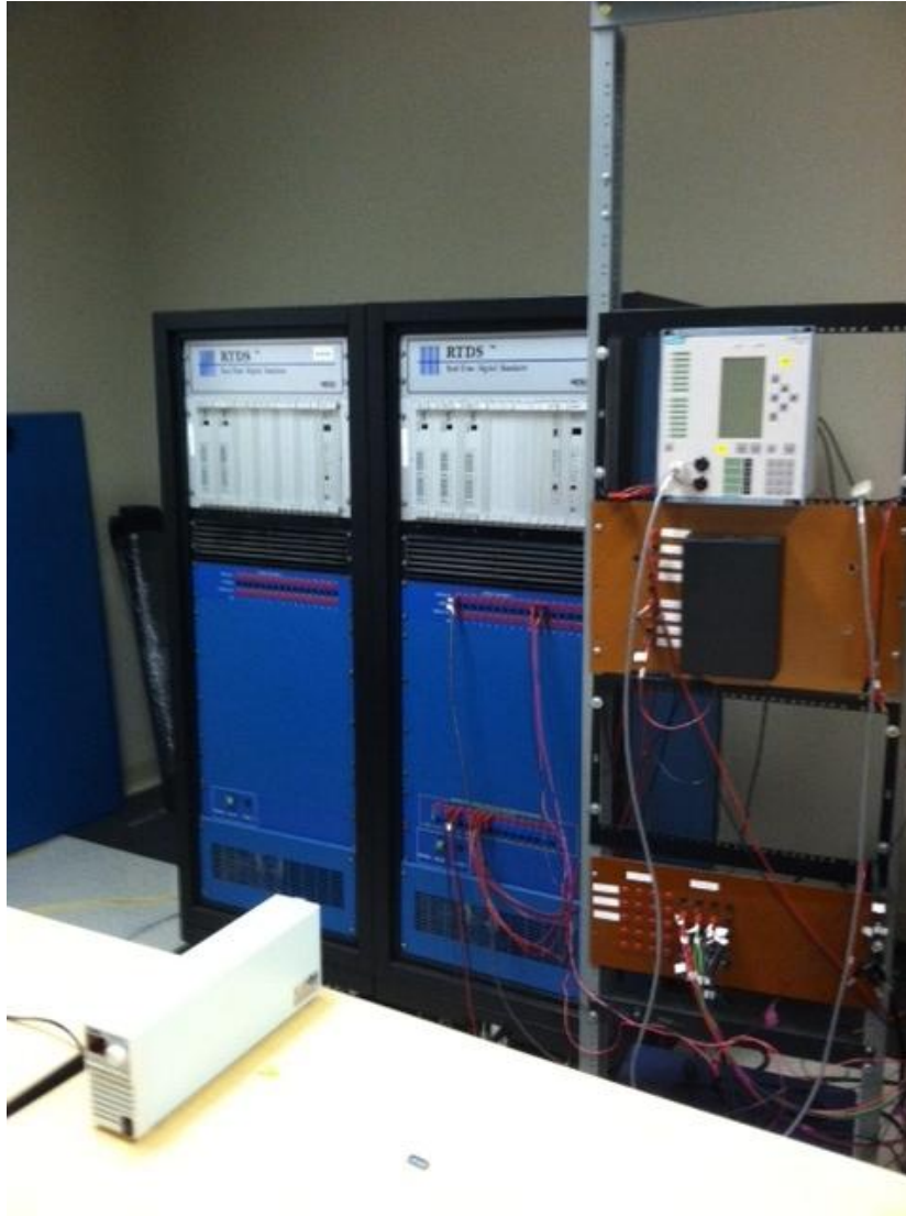
Figure 2-21. Real Time Digital Simulator (RTDS) facility at FREEDM Systems Center.
