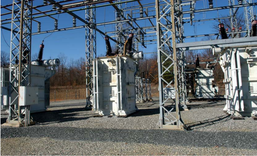
Fig. 2.5 Duke Energy substation
