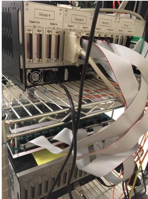
Figure 6.7: Fault-tolerant Controller in Connection with Opal-rt System (back view)
