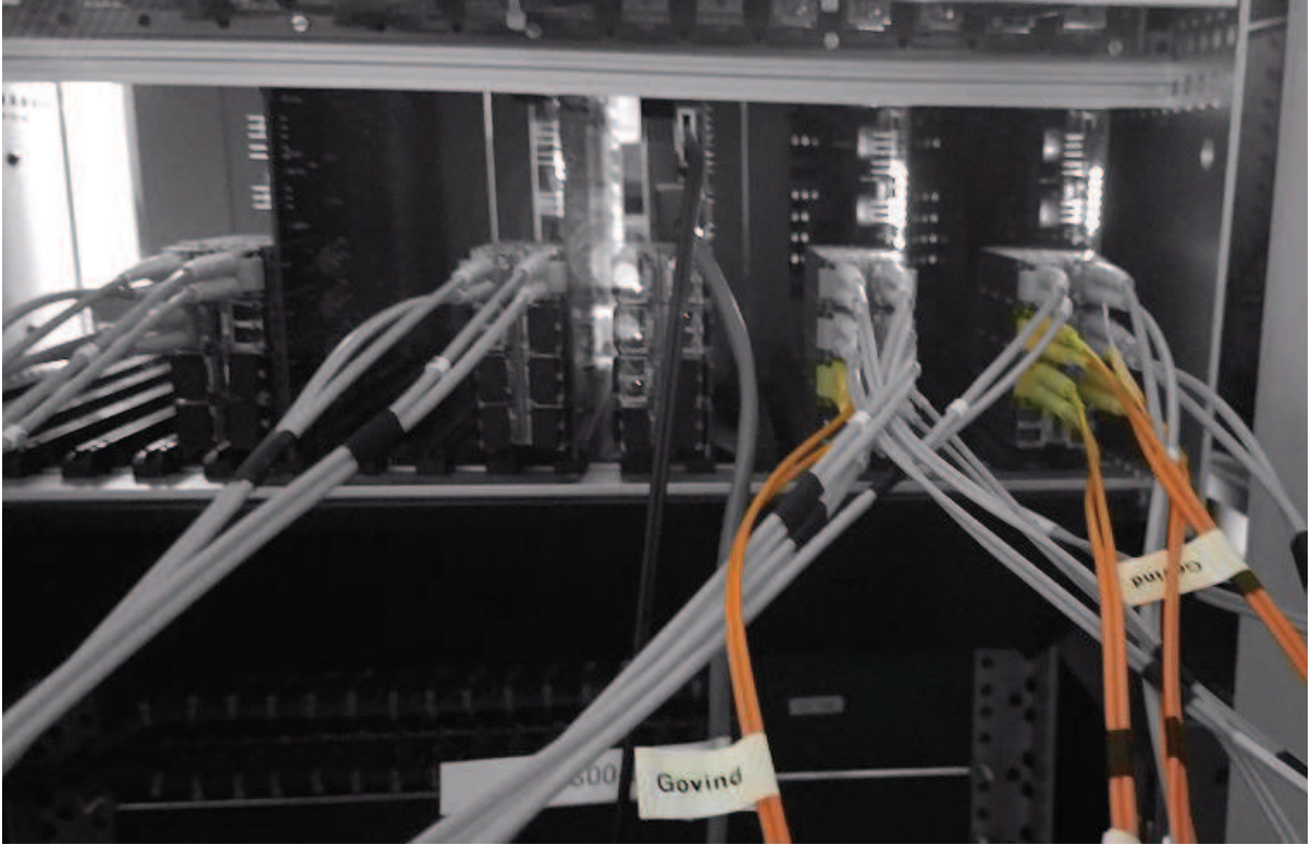
Figure 5.18: Back-plane interconnection between RTDS cards for ‘small-dt’ communication using optical fibers
