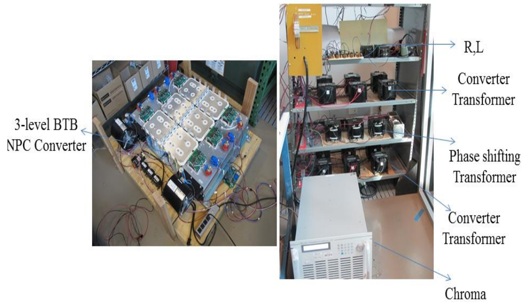
Figure 6-33. Experimental test-bed for Active Mobile Substation based on 3-level NPC converter.
